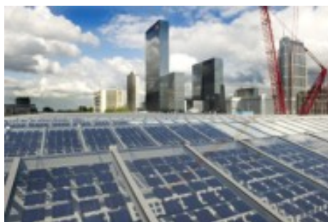
出展：RCI HP-The solar panel roof on Central station
